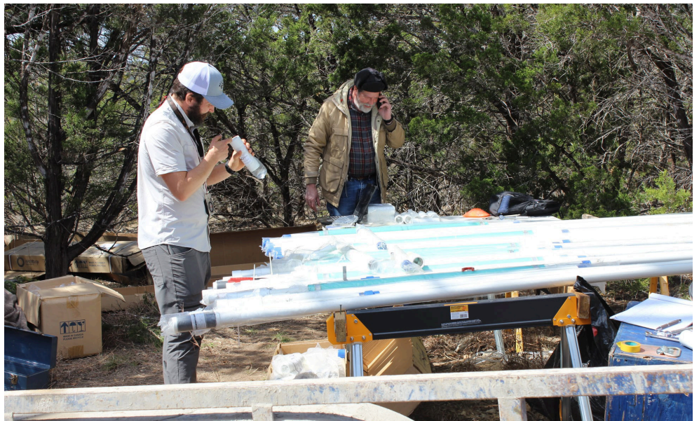
BSEACD Senior Hydrologist Brian Smith and Staff Hydrologist Jeff Watson oversee drilling and monitoring of the well.
