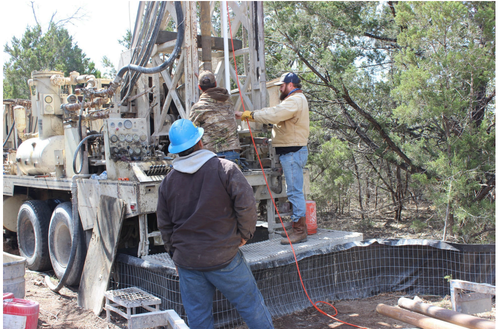
TGWA members GEO Projects drilled the monitoring well and Well-Scope logged the well.
