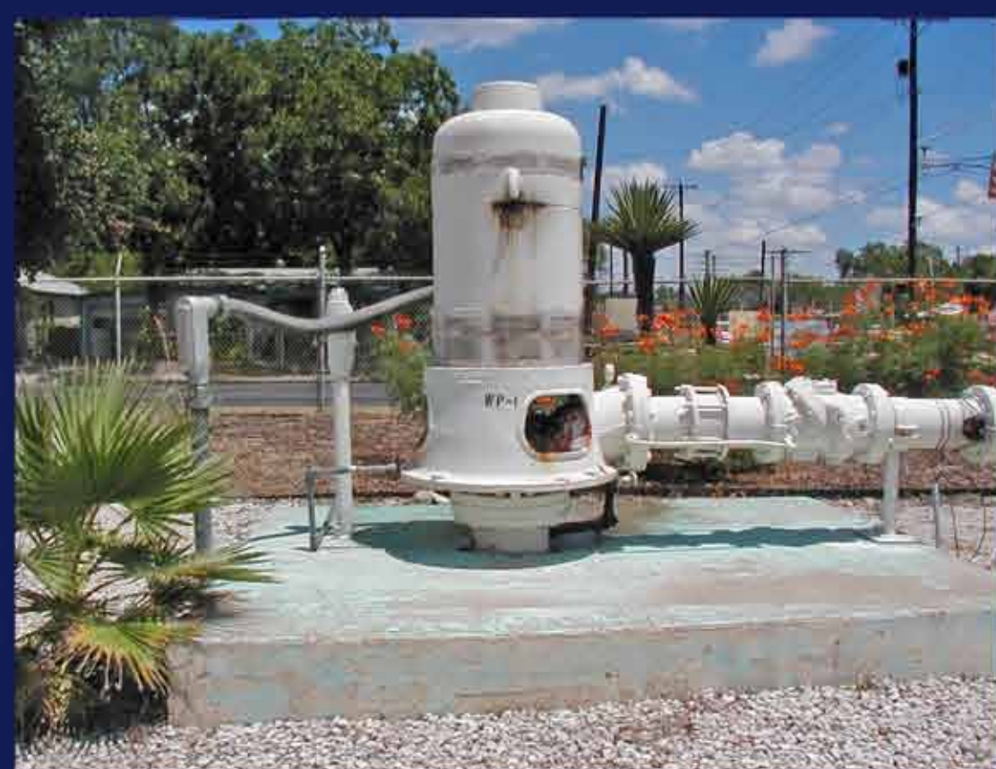
A public water supply wellhead in San Antonio, TX
